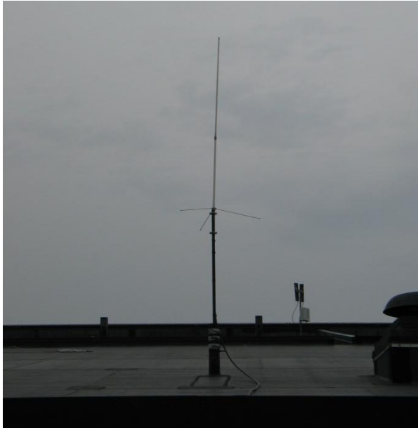
Figure 1 - The roof-mounted 145.31 antenna
